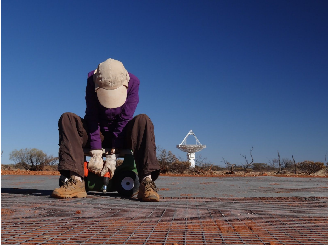
Figure 5. Using a brush head on a power screwdriver to clean the welds before spraying with zinc sealer.
