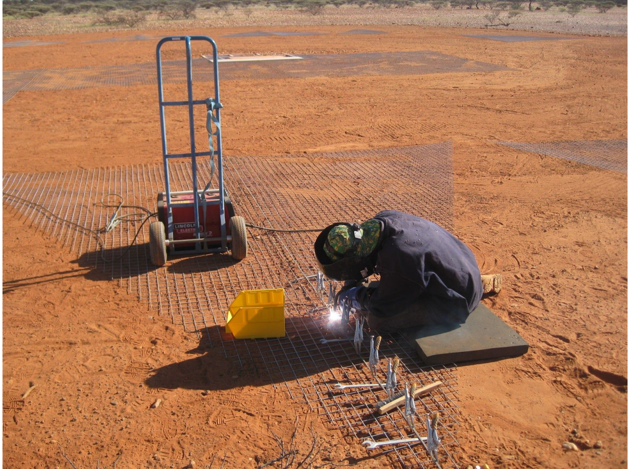
Figure 3. Showing use of crescent wrenches to prop up the mesh for welding.
