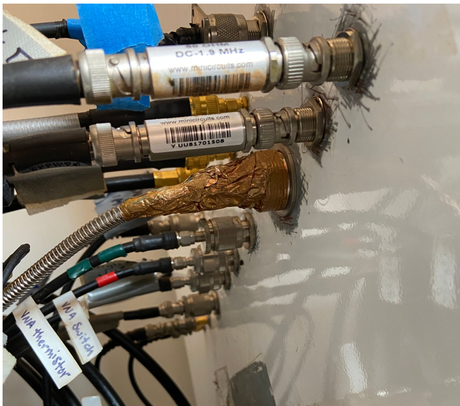
Row-2 Outside cabinet
