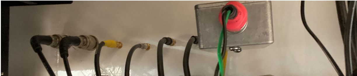
Row-1 Inside cabinet
