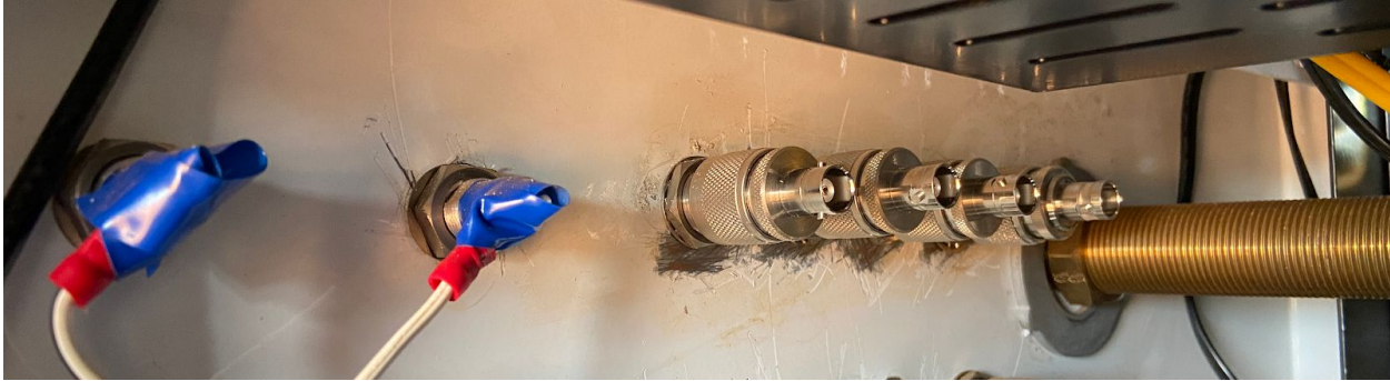
Row-3 Inside cabinet
